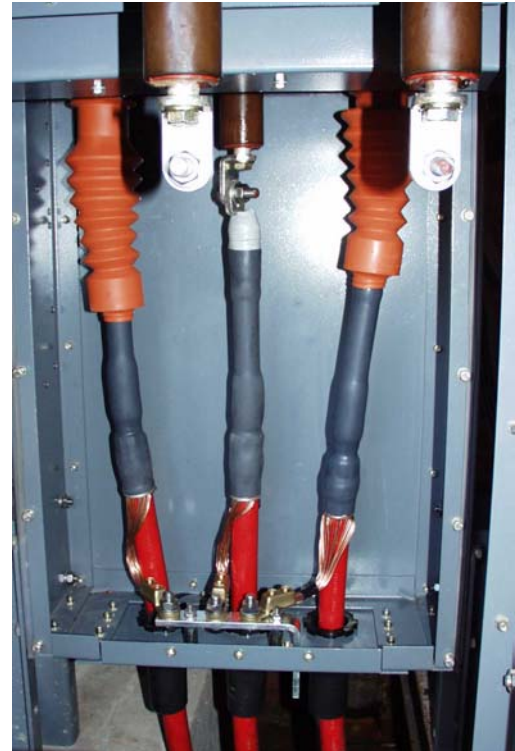
single core switchgear termination
