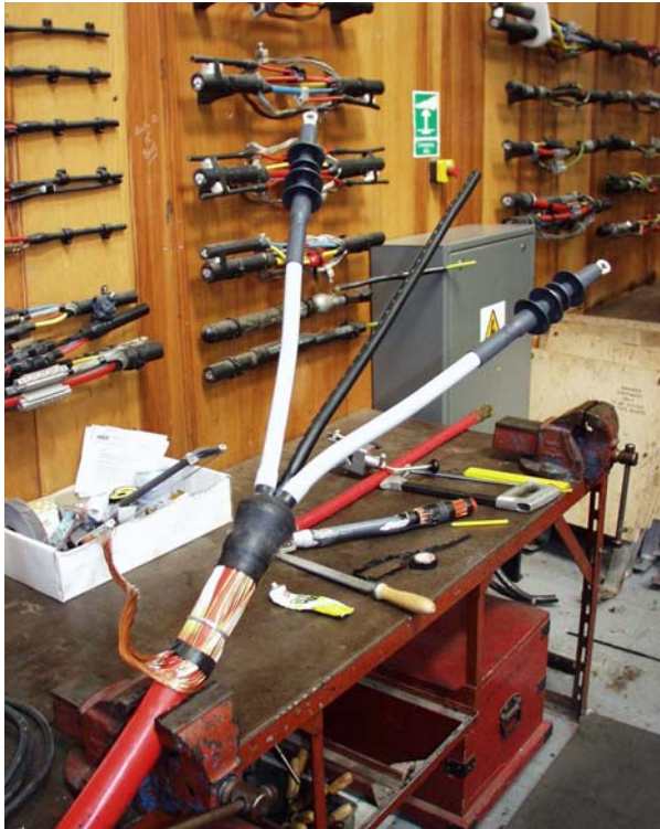
3 core overhead termination
